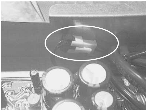
Figure 7 – Evaporator Thermistor Connection (inside power supply)
